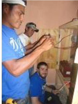
2014 Wiring up the Batteries
