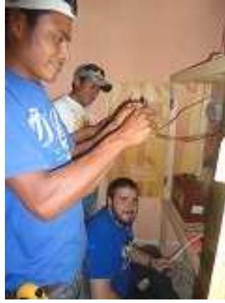
2014 Wiring up the Batteries
